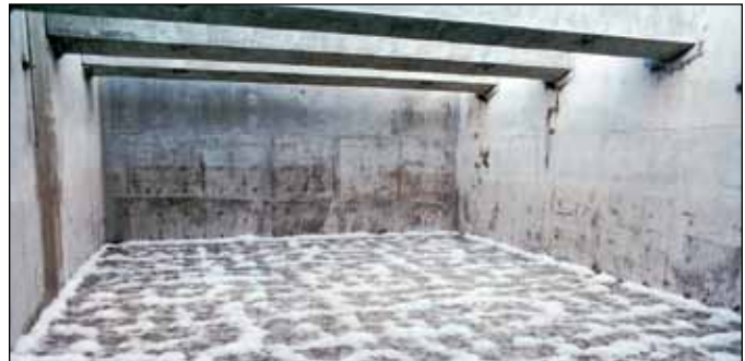
Better air scour action – and better media cleaning – is the result of closely spaced, non-clogging orifices and uniform distribution of air throughout the length of the underdrain lateral.
